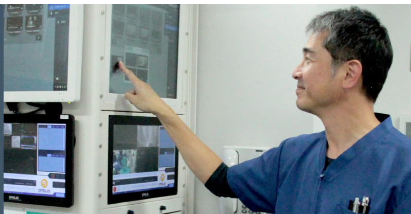
Ichinomiya Municipal Hospital uses Getinge’s Tegrís OR integration system to connect 15 rooms, including 12 operating rooms, two cath labs and a hybrid operating room.
